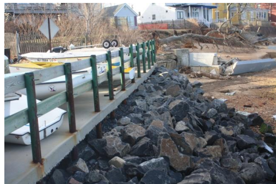
Figure 9: This slab at the KYC was undermined by erosion and the rip-rap projection was compromised by storm surge erosion and settlement, with some scattering of smaller rock by Sandy.
