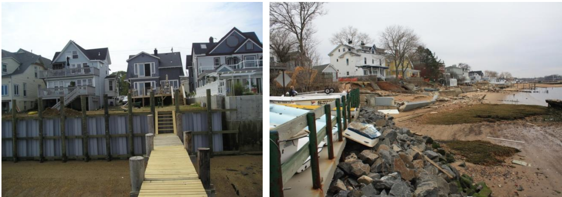
Figure 8: (Left): Bulkhead photo at 51 First Street after Superstorm Sandy, which pushed water to an elevation of ~ 14 ft. The new bulkhead is ~9 feet in height above the beach, which gives it a flood elevation of ~ 13 feet. Courtesy of Michael Lane, Keyport, NJ (Right) Damage to bulkheads along First Street facing west from Keyport Yacht Club in April, 2013 Courtesy of Maser Consulting, PA
